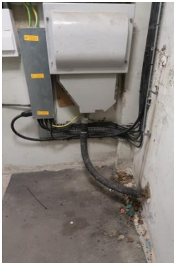
Incoming Service Head
