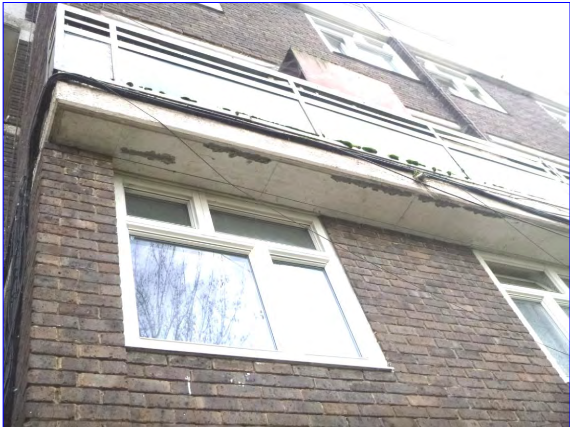
Photograph 18: Spalls noted to slab soffit on Heversham House.
