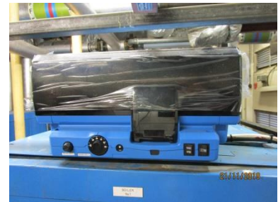
New Boiler Controller
