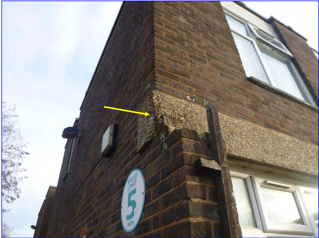
Photograph 10: Spalling to a corner, Manor Grove.
