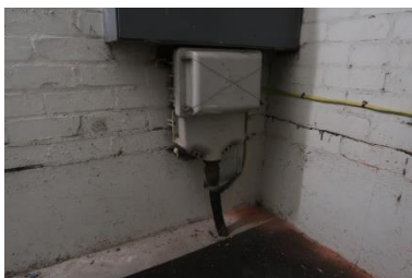
Incoming Service Head
