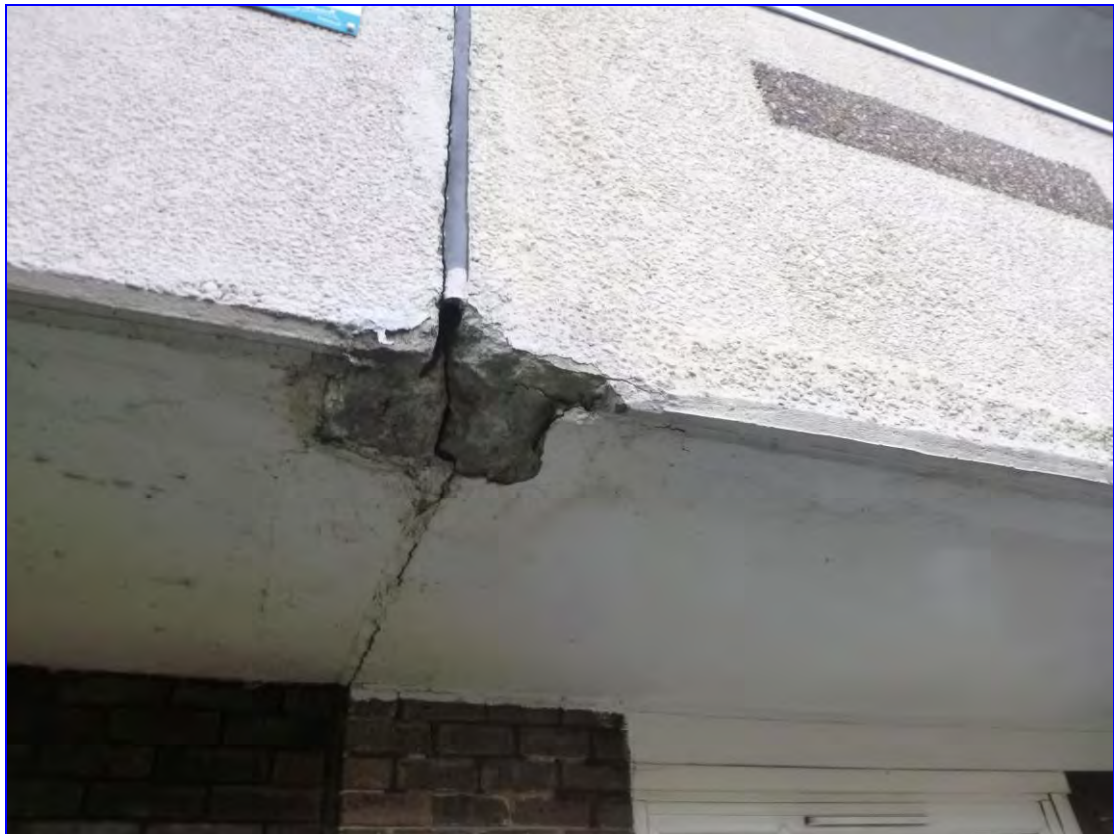
Photograph 16: Further example of deterioration on Kentmere House.
