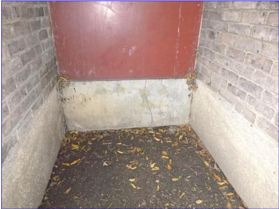
Photograph 26: Cracking to floor beam on Ullswater House.
