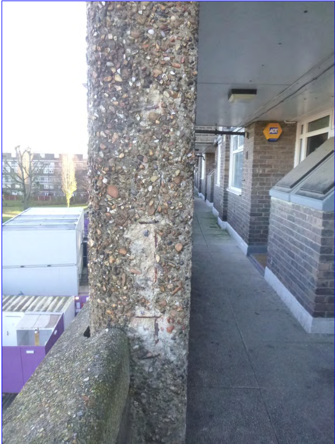
Photograph 25: Another example of spalling, here to a column on Bowness House, at TA38.
