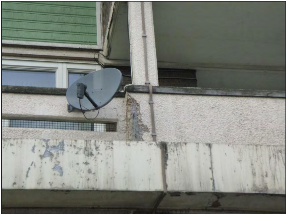
Photograph 20: Another example of spalling to Heversham House.
