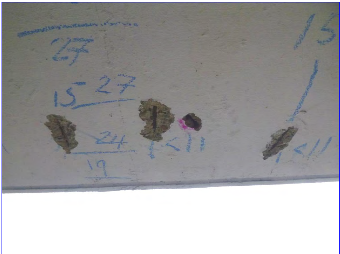
Photograph 14: As photo 13 after spalling material removed at the test area.
