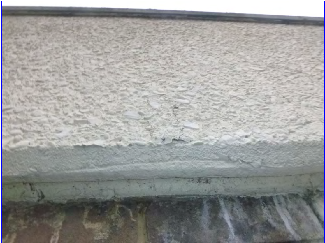
Photograph 11: Spalling to roof beam on Kentmere House.
