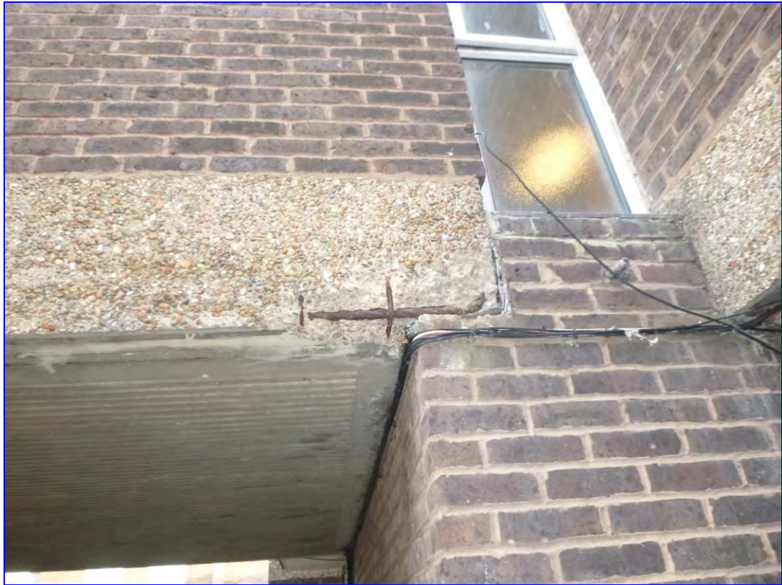
Photograph 8: Another example of a spall to Manor Grove.
