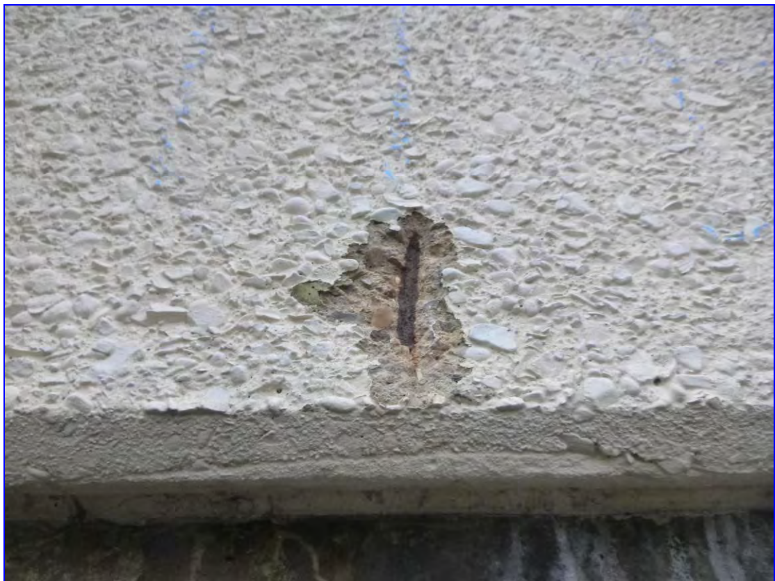
Photograph 12: As photo 11, after spalling material removed revealing corroded rebar.
