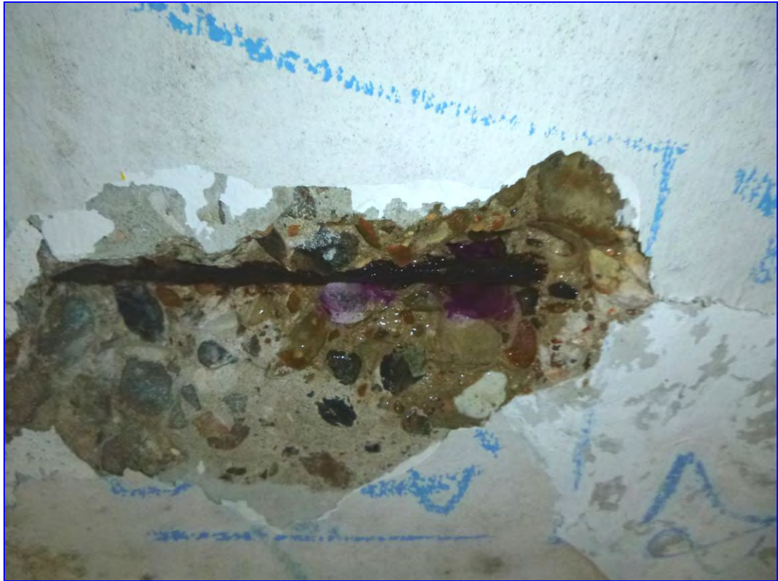
Photograph 34: The breakout at TA54, soffit, Kentmere House, revealing a bar with surface corrosion/loss of section in carbonated concrete.
