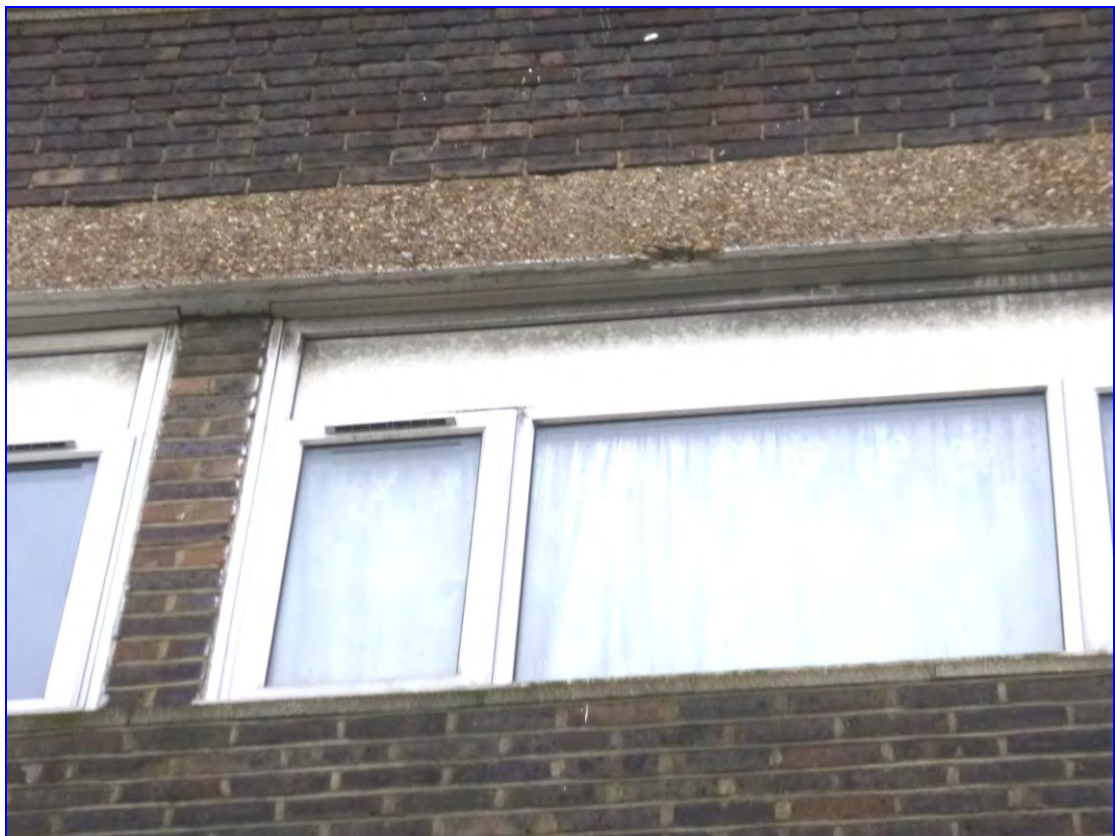
Photograph 23: A spall to a beam over a window, Bowness House.
