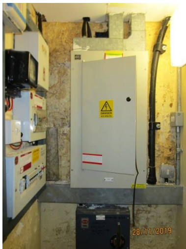
Older Distribution Board
