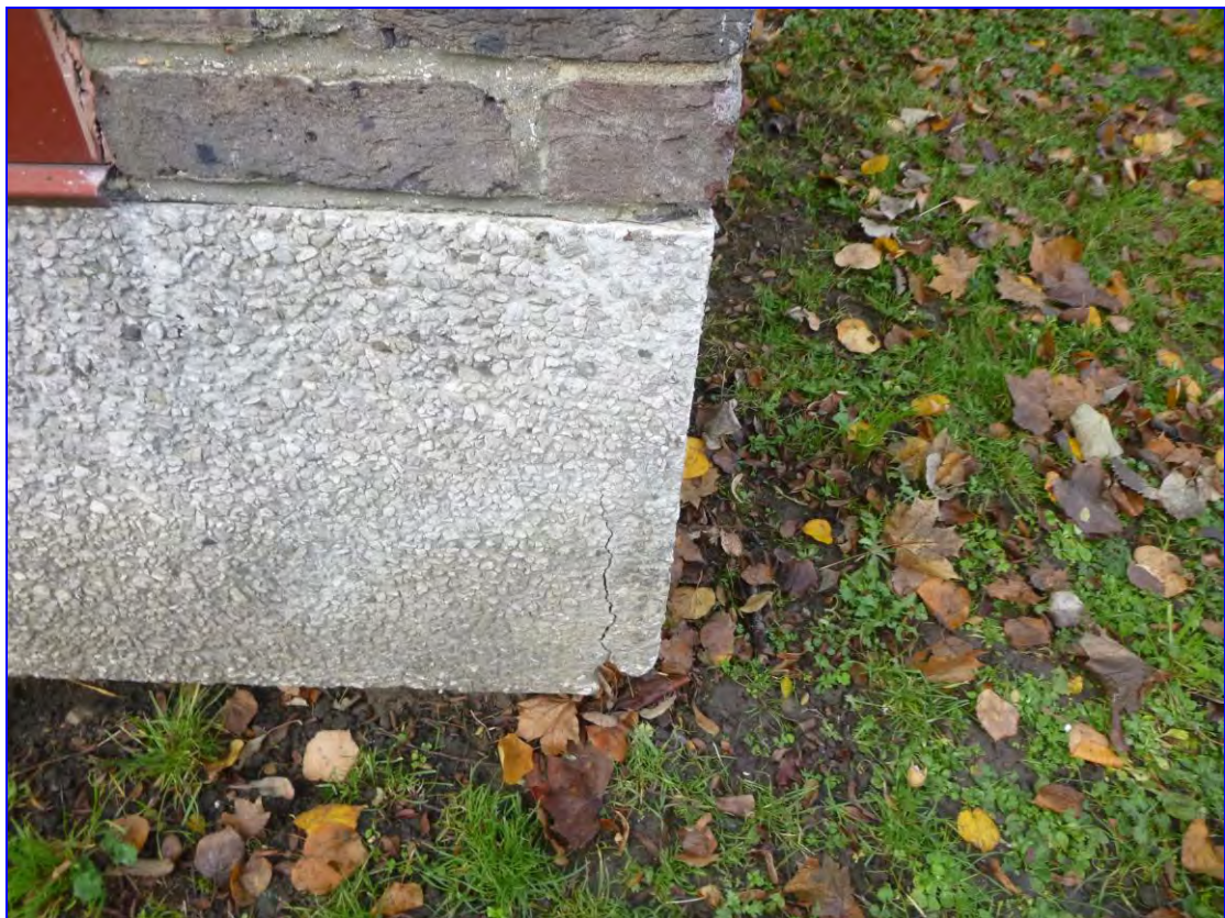
Photograph 27: A spall to a corner, pc panel, Ullswater House.
