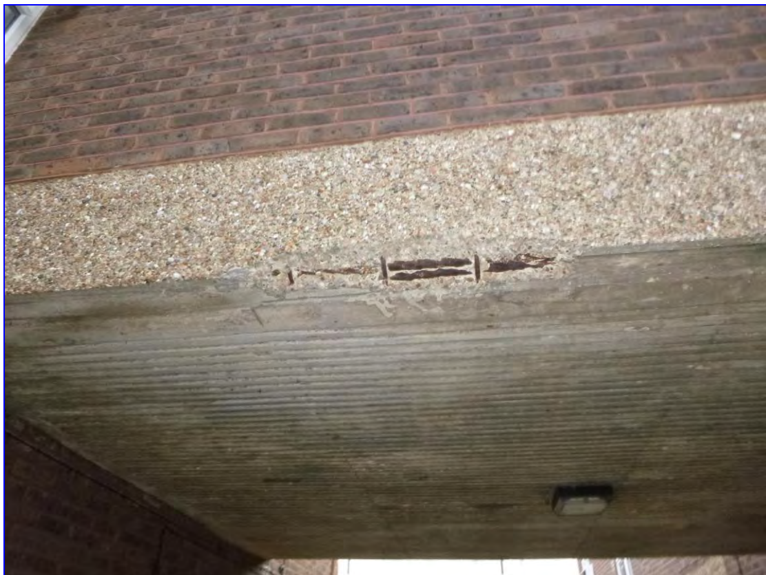
Photograph 7: Example of spalling and visible reinforcement on Manor Grove, to a link section.
