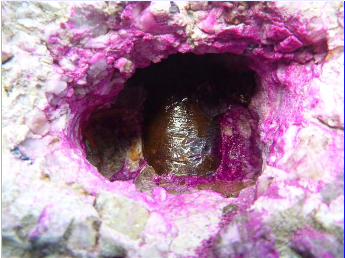
Photograph 31: The breakout at TA7, pc panel, Ullswater House, revealing a bar with slight surface corrosion where carbonation had reached the bar down a crack (central to this photo).
