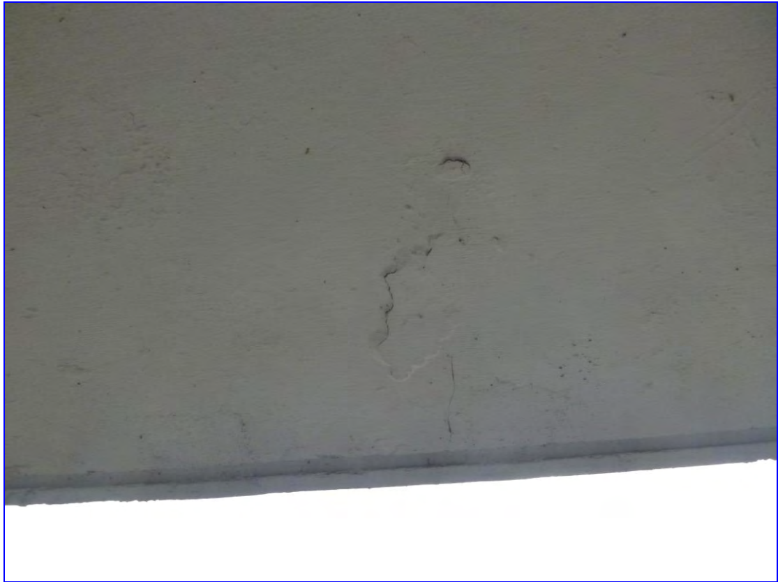
Photograph 13: Spalling to soffit, Kentmere House, at TA52.
