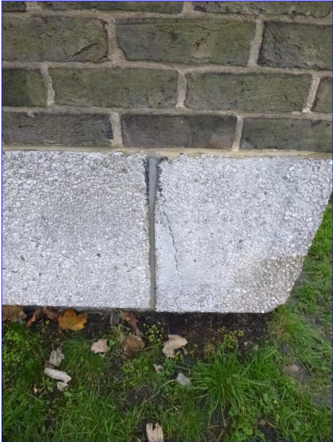
Photograph 28: Spalling to a pc panel at a joint, Hill Beck House.
