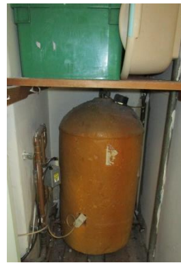
Hot Water Cylinder and Header Tank
