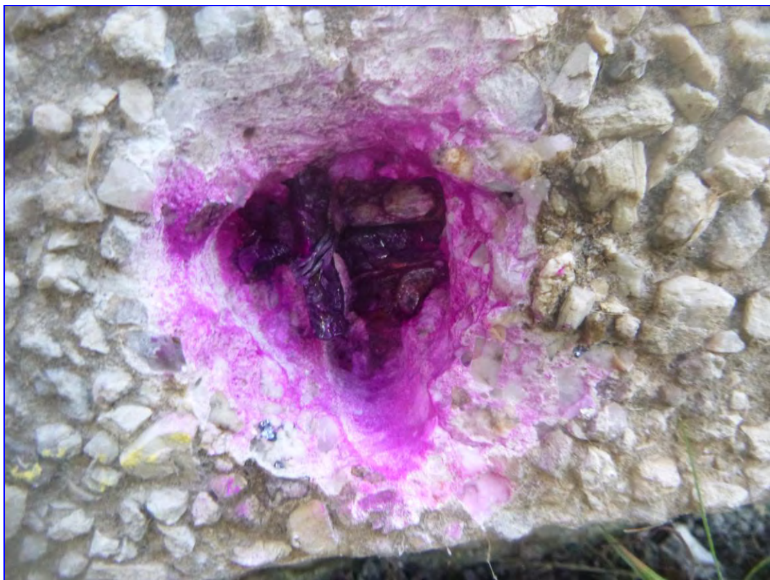
Photograph 30: The breakout at TA1, pc panel, Hill Beck House, revealing clean and passive reinforcement in alkaline concrete.
