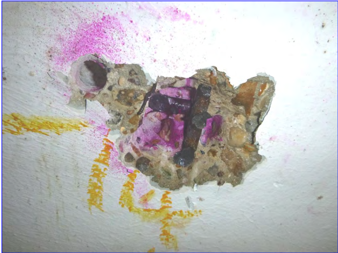
Photograph 32: The breakout at TA24, soffit, Heversham House, revealing one bar in carbonated concrete with slight surface corrosion and a bar at deeper depth in alkaline concrete and clean and passive condition.
