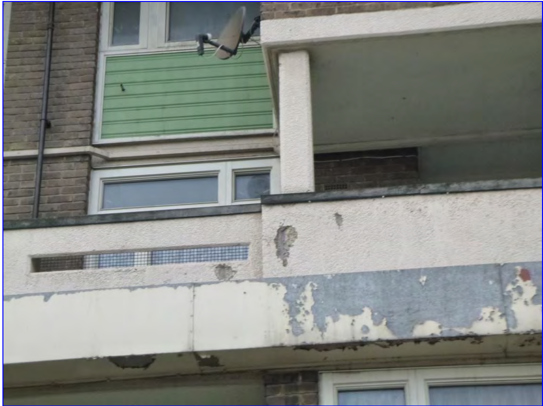
Photograph 19: Further spalling to Heversham House, with exposed rebars at spalls covered with a grey primer.
