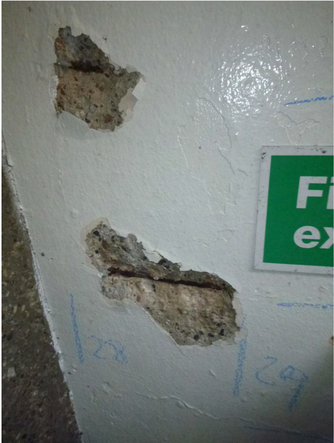
Photograph 21: Spalling to stair tower roof at TA42, on Bowness House.
