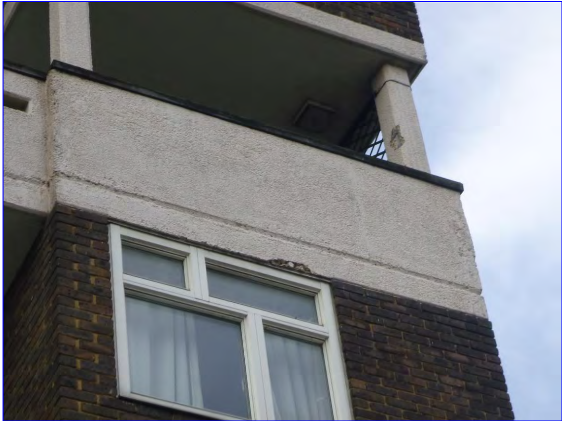
Photograph 17: Example of spalls to Heversham House, here to window head and column above.
