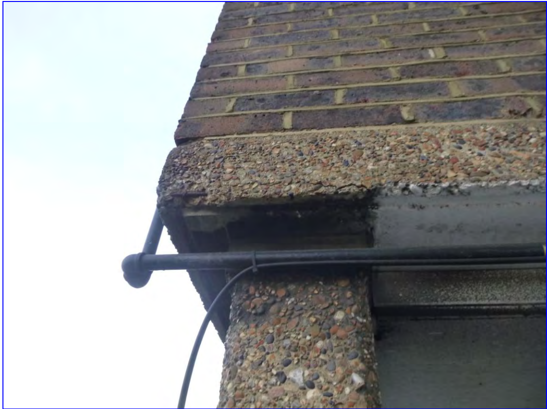
Photograph 24: Spalling and visible rebar on Bowness House.
