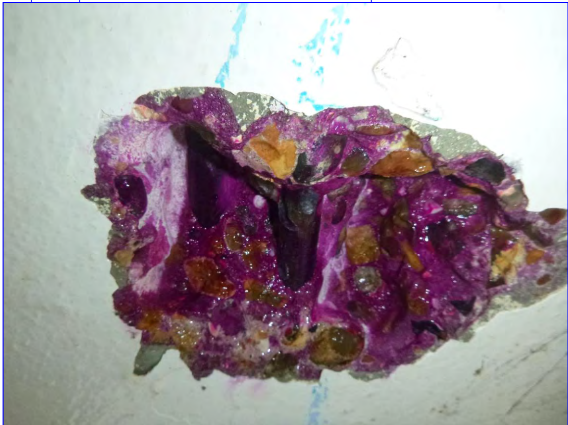
Photograph 33: The breakout at TA37, soffit, Bowness House, revealing clean and passive rebar in alkaline concrete.
