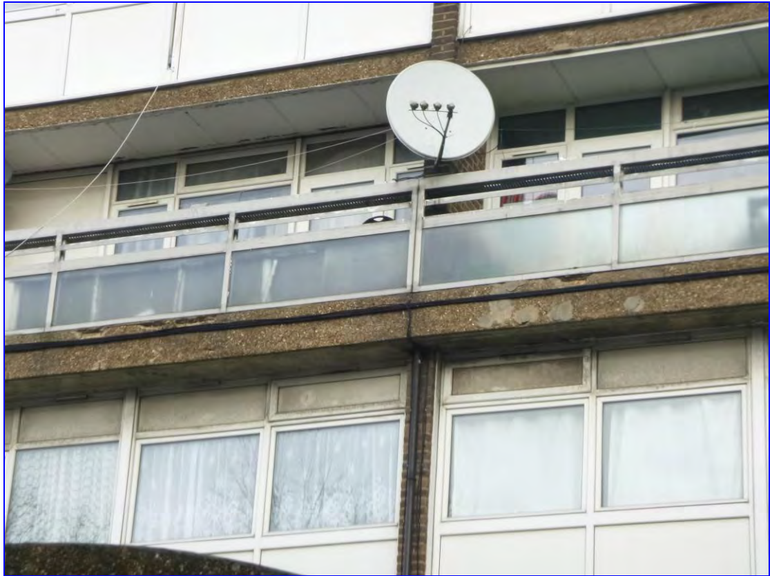
Photograph 22: Example of various spalls and previous repairs along floor beam, Bowness House.
