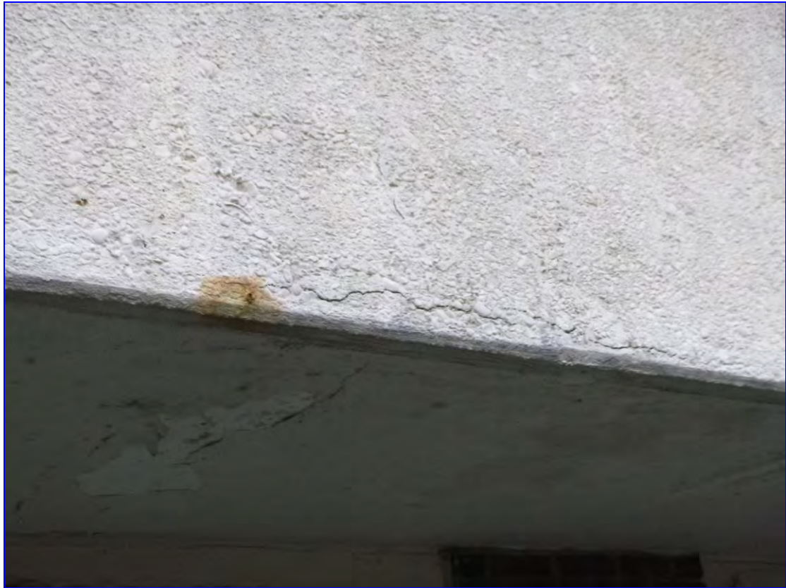
Photograph 15: Another example of spalling on Kentmere House. Also note deteriorated paint coatings to soffit.
