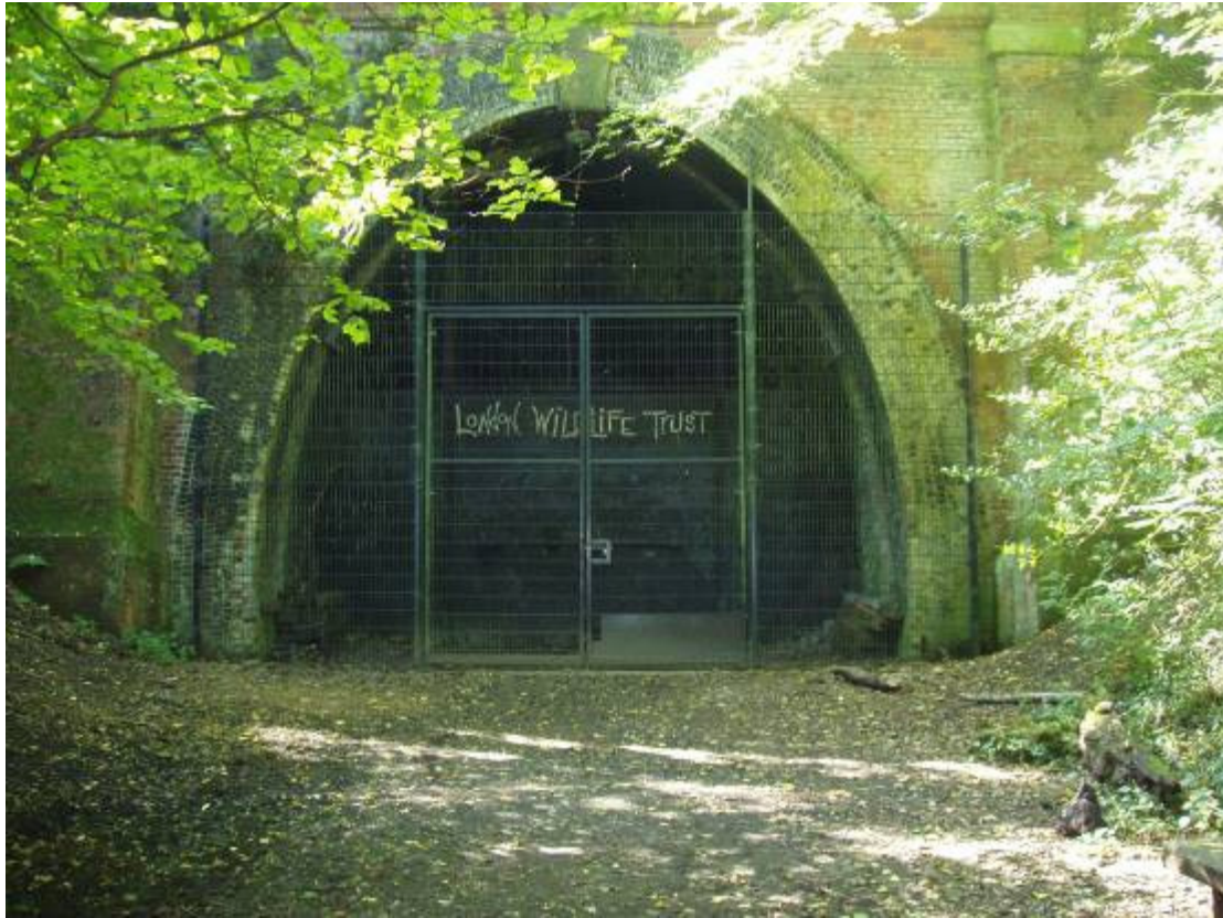
Entrance to the railway tunnel in Sydenham Hill Wood LNR (Now a registered bat roost).
