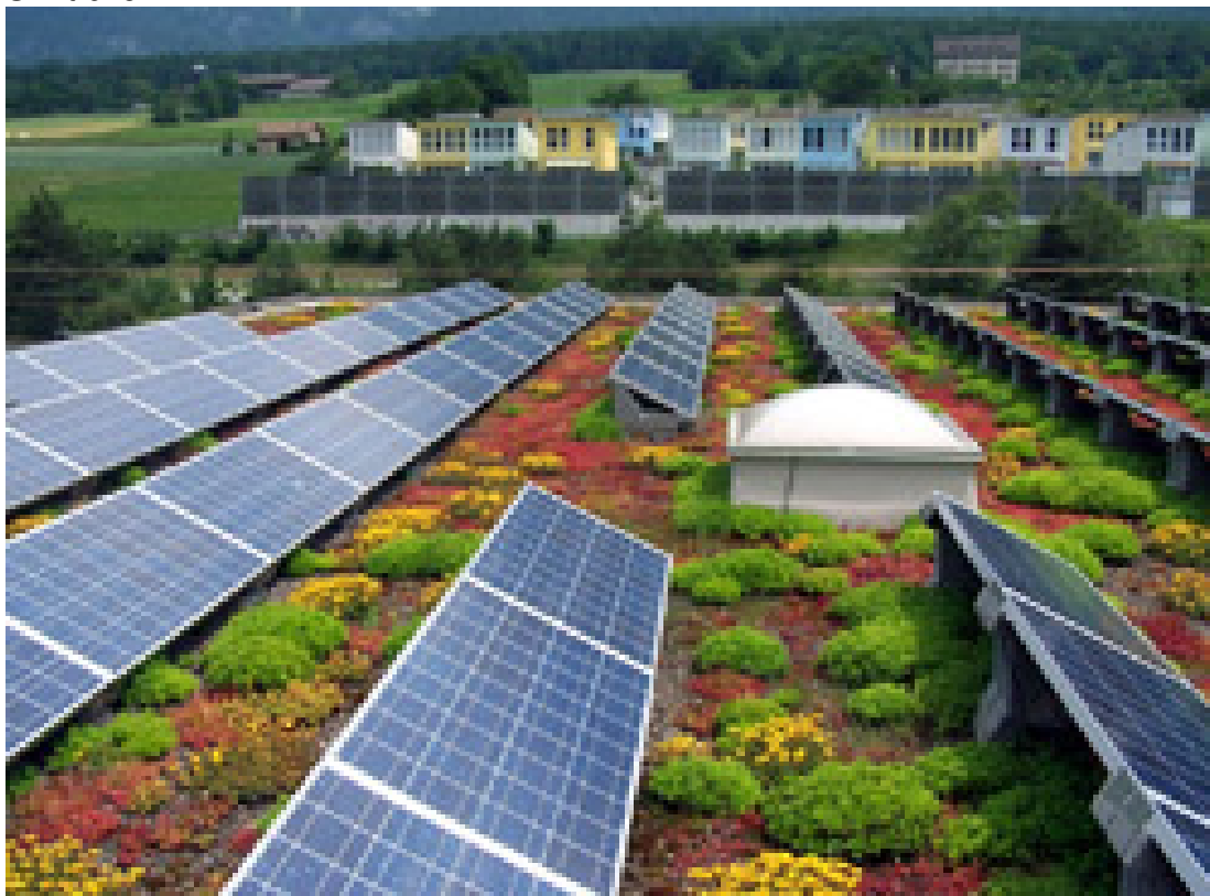
Sedum roof with Photo voltaic panels
