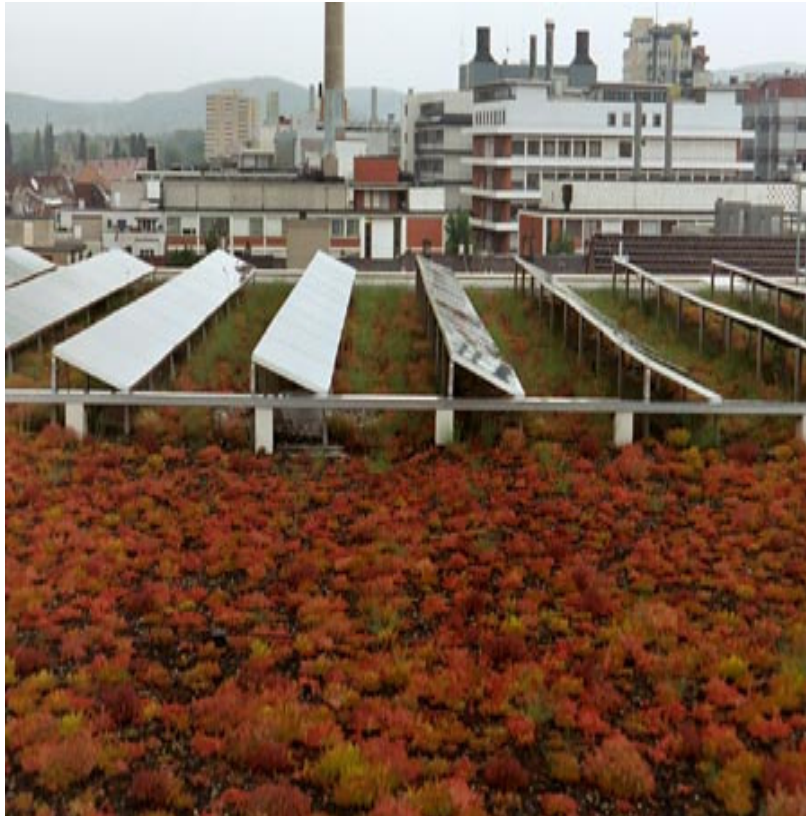
Brown roof with photo voltaic panels
