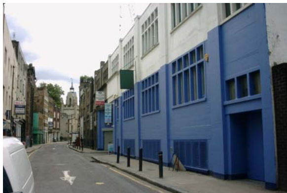
Figure 22 Looking south to St. Mary Magdalene, showing concrete buildings at 156-170 Bermondsey Street, with repaired and painted façades.
