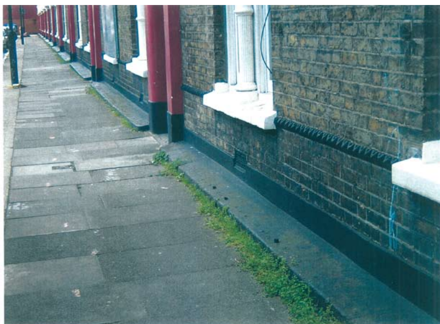
Figure 9: The pavement in Iliffe Street, showing the stubs of the removed railings.
