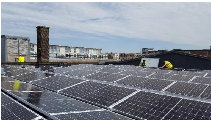
Solar panels at Walworth Methodist Church
