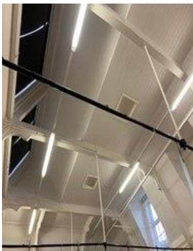
The roof of a hall at Goodrich Primary School with new lighting
