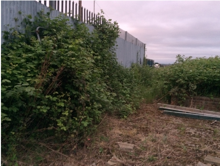
Photograph 11 (TN13): Brambles have colonised around parts of the security fencing
