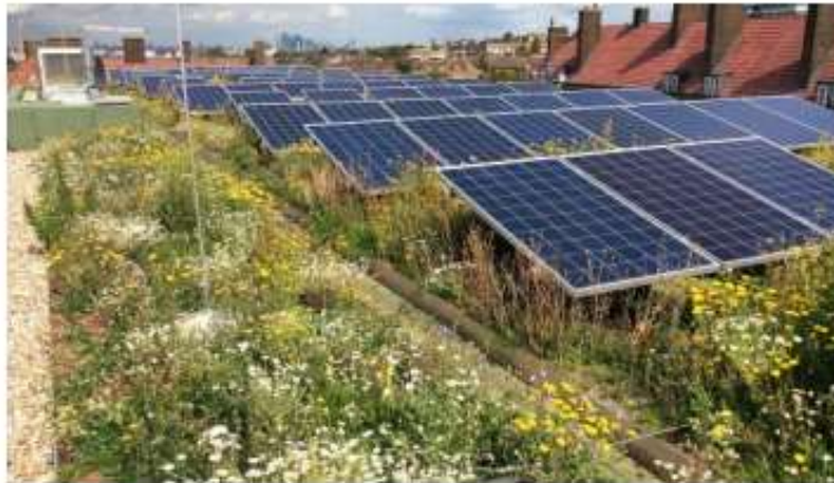
Biosolar roof, Clapham Park, Lambeth, London Photo: Bauder
