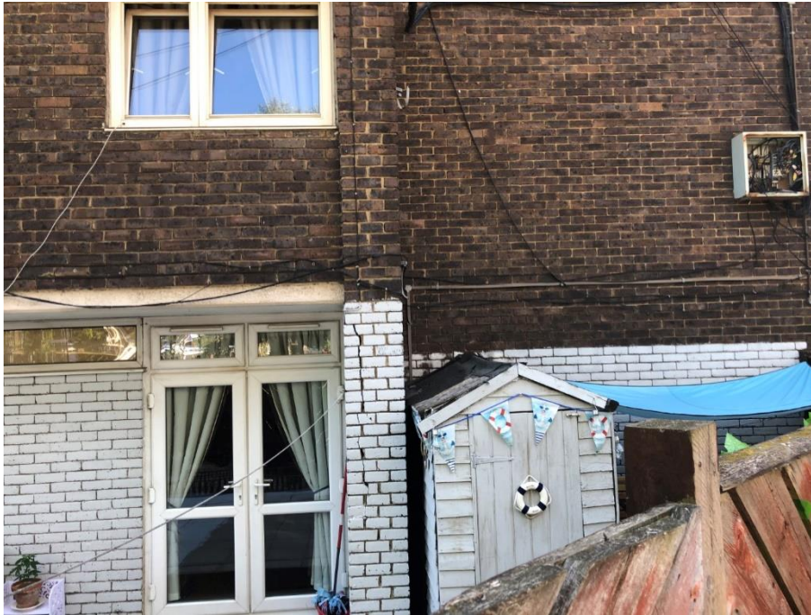
Photograph 3 – Heversham House – Vertical cracking through brickwork nibs.
