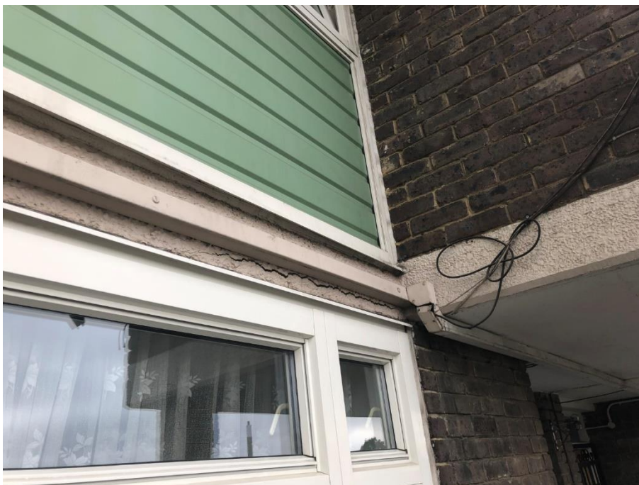
Photograph 2 – Heversham House – Spalling to downstand beams over window openings.
