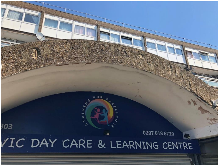
Photograph 8 – Bowness House – Spalling to slender concrete upstand to shop front canopies.
