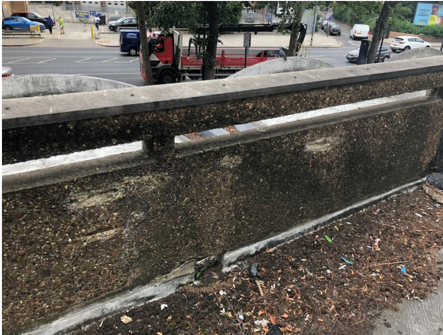
Photograph 7 – Bowness House – Spalling to rear face of parapet over shop fronts.
