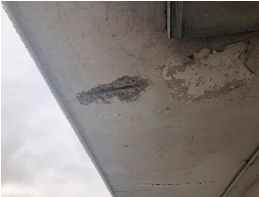
Photograph 1 – Heversham House – spalling to soffits.
