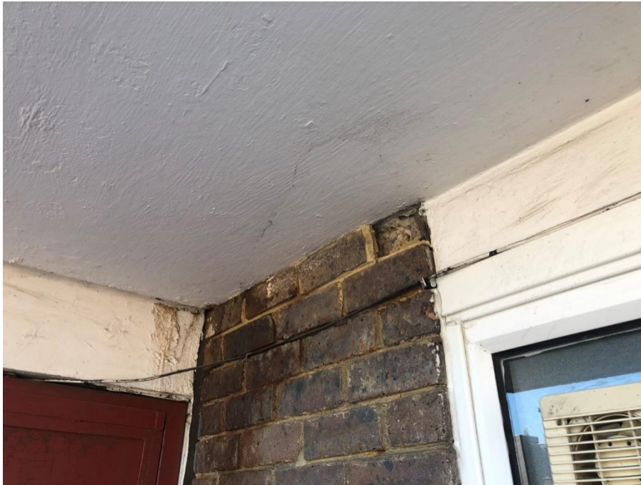
Photograph 5 – Kentmere House – Damage to slip bricks.
