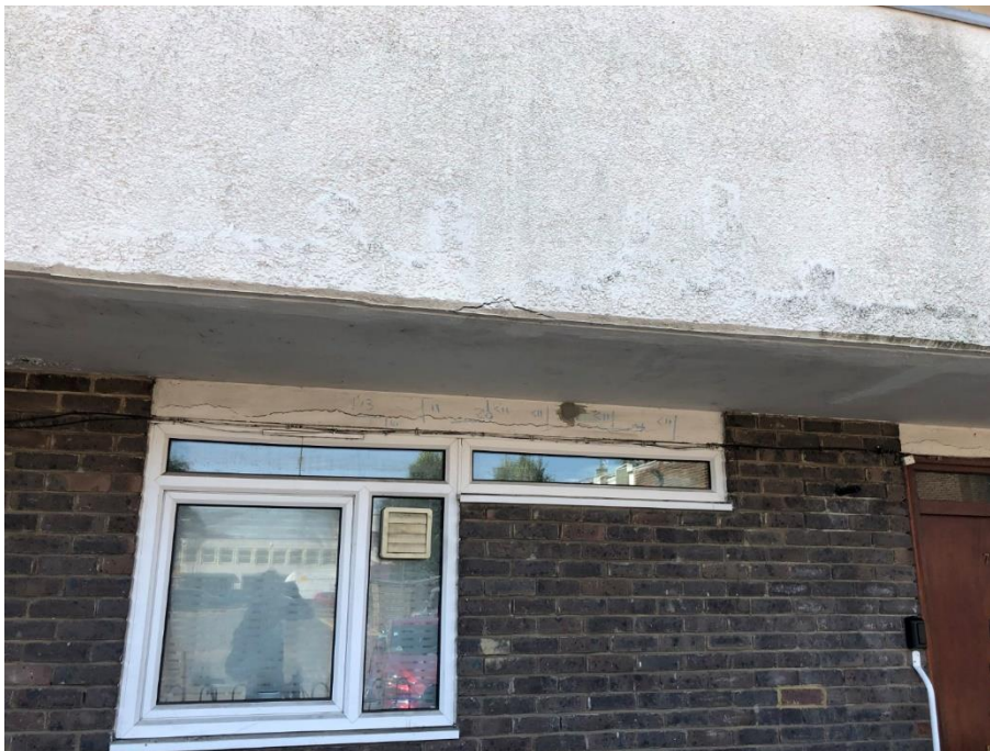
Photograph 4 – Kentmere House – Spalling to downstand beams over window openings.
