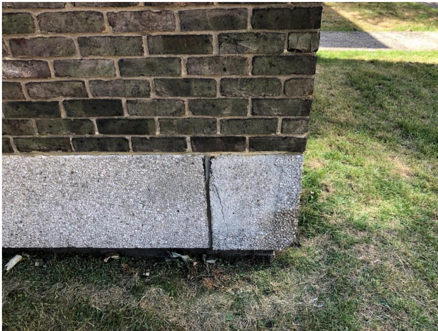
Photograph 10 – Typical concrete defect at Ullswater House and Hill Beck Close.
