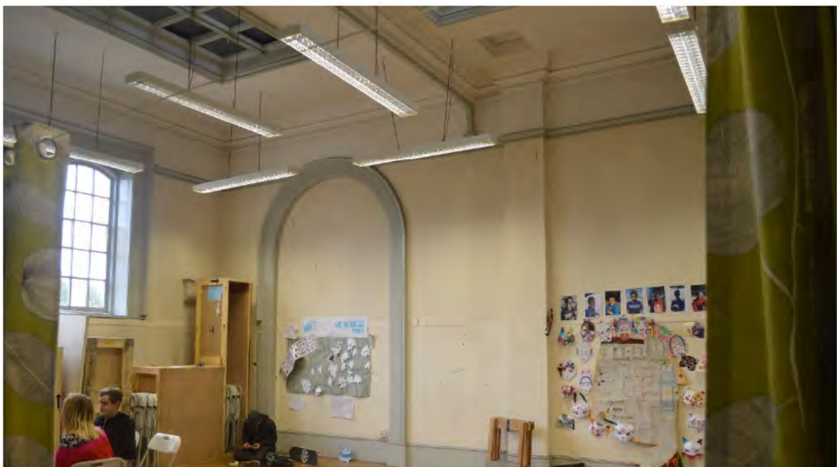
Present interior of former library with blind arch in north east corner (offering potential for an opening giving equal access from the park)
