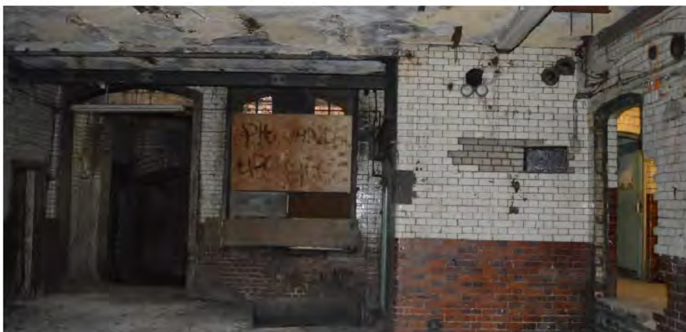
Basement area showing robust character of the spaces with tiles walls and internal windows
