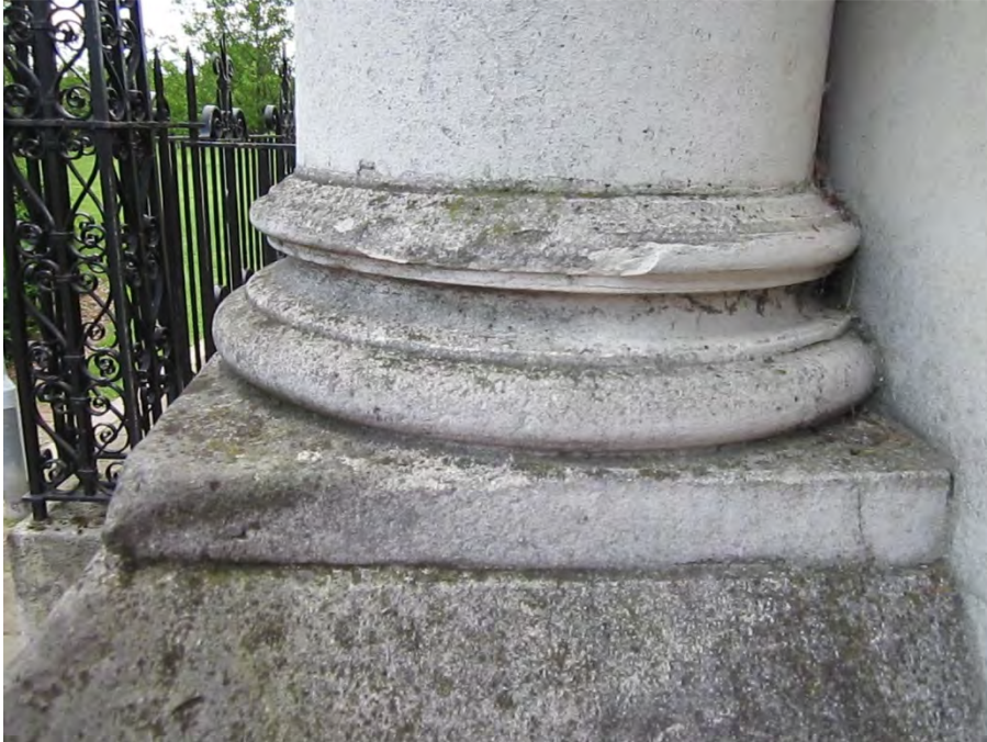
3 DAMAGE TO PORTLAND STONE PILLARS TO FRONT ENTRANCE
