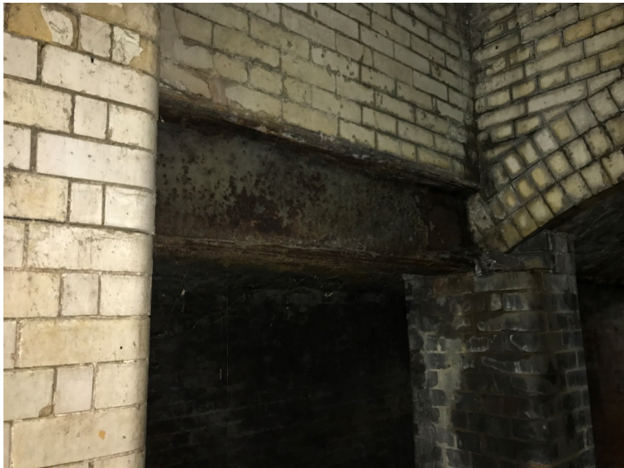
16. Heavily Corroded Steel Beam
