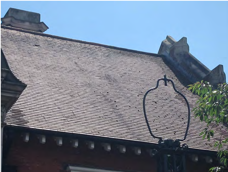
1 VIEW SHOWING SLIPPED AND MISSING TILES TO ROOF
