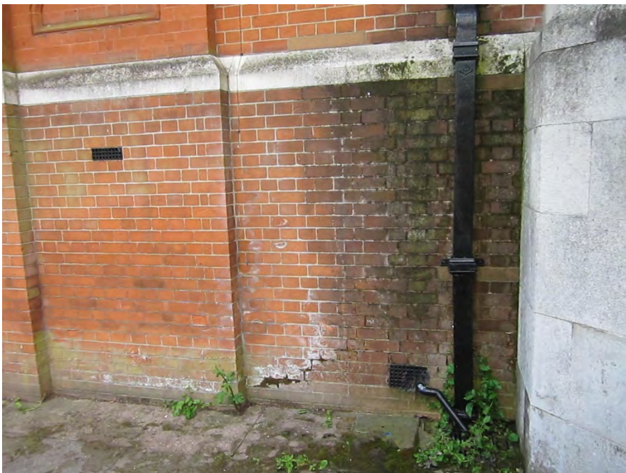
2 BRICKWORK STAINING TO LEFT-HAND SIDE OF ENTRANCE TO NORTHERN ELEVATION
