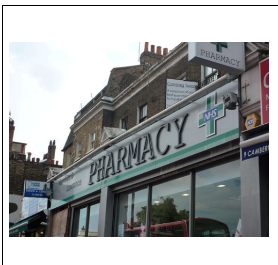
Camberwell Road: Inappropriate modern fascias can detract from the overall quality of a building
