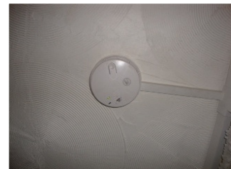
Mains Smoke Detector
