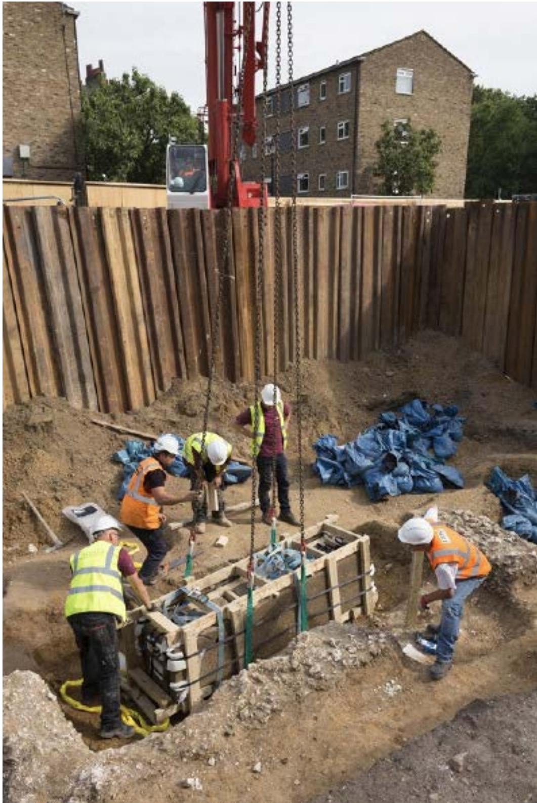
The main excavation area at Harper Road, Borough where a Roman sarcophagus and Roman buildings flanking the realigned course of the Roman road of Stane Street were discovered
