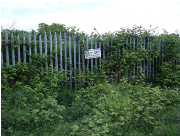
The security fencing is in a good condition but is a harsh feature within the landscape.
