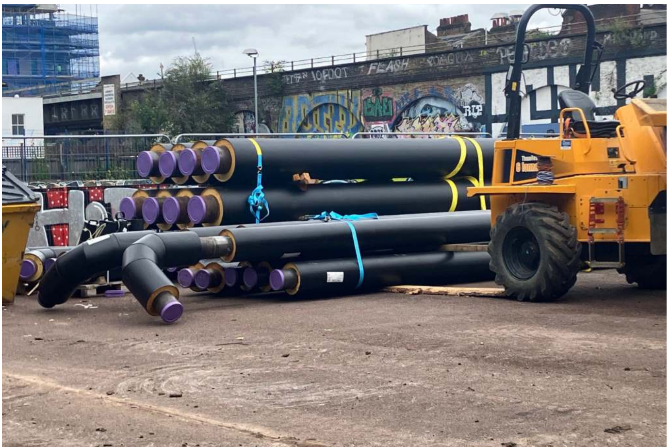
District Heat Network pipes on site at Brimington Park prior to installation
