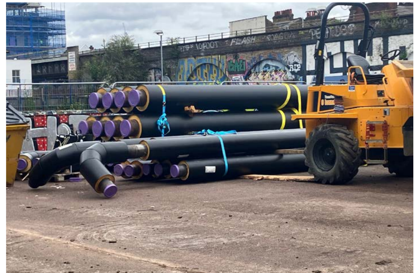
District Heat Network pipes on site at Brimmington Park prior to installation
